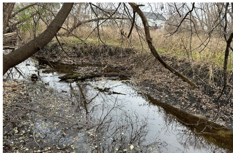
A section of eroding streambank along ǪǪǪ Wakpádaŋ / Main Stem of Bassett Creek evaluated in 2023 (Photo: Barr Engineering Co.).
