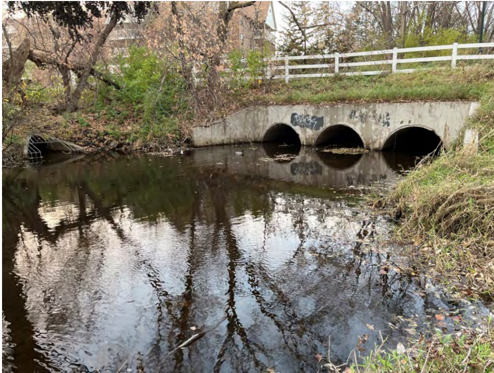
Photo 42: Site 4g. Looking upstream at station 69+00 towards the 38th Avenue crossing. Slight sediment build up in center of channel near the culverts.
