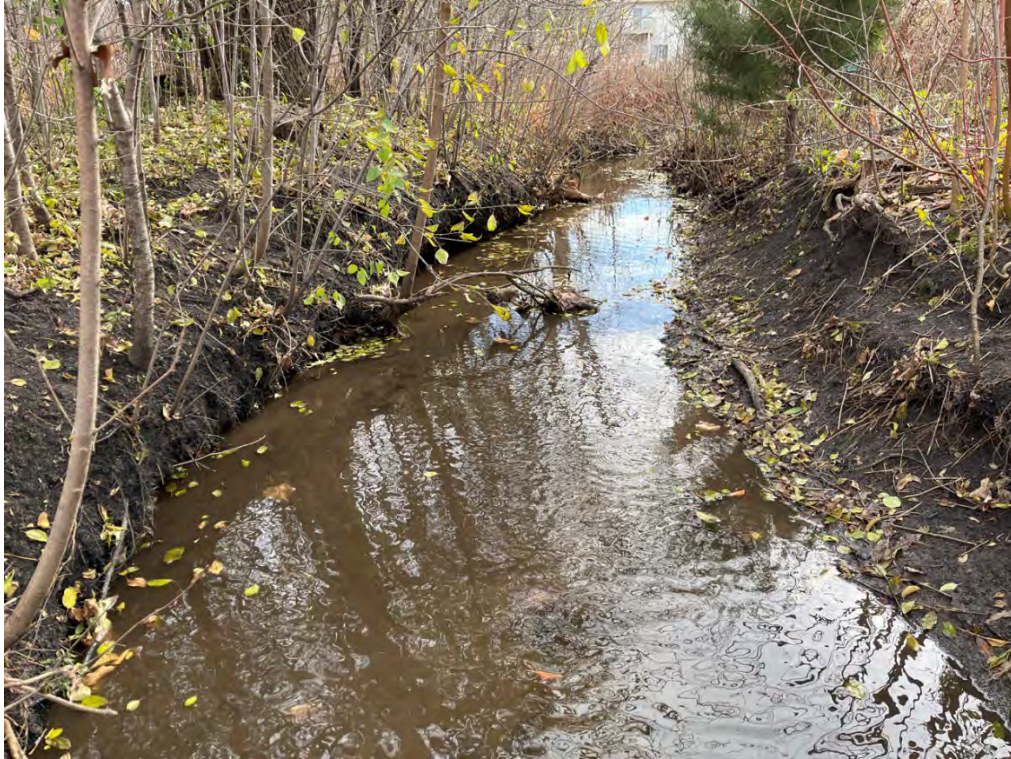
Photo 5: Site 1c. Looking downstream at station 6+40, slight undercut for left bank and slumping on the right bank.
