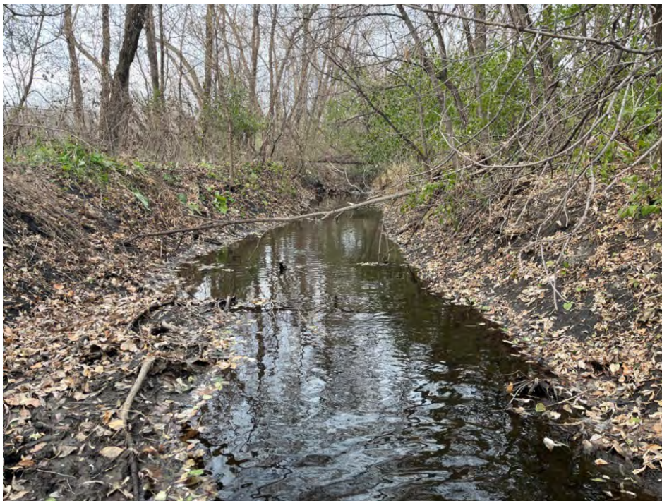
Photo 21: Site 2d. Looking upstream at station 26+50, both banks are angled at approximately 60 degrees and are bare.
