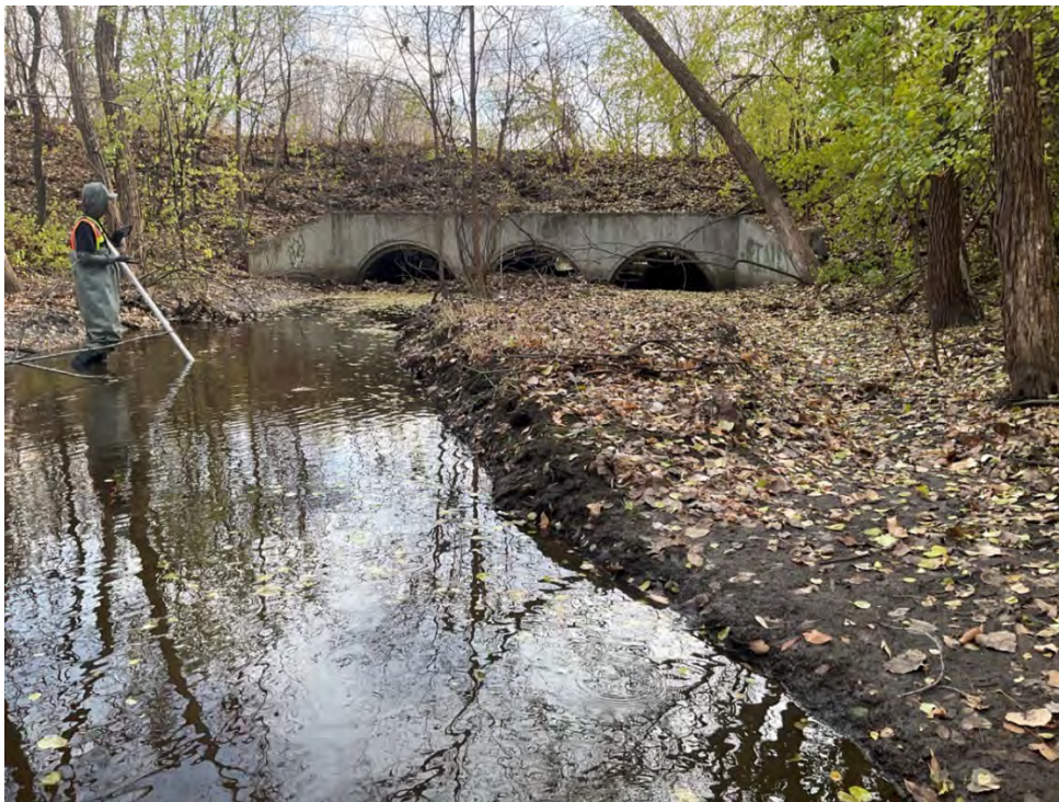
Photo 41: Site 4f. Looking downstream at station 66+90 towards the 38th Avenue crossing. The center and right culvert are partially blocked by sediment deposition.
