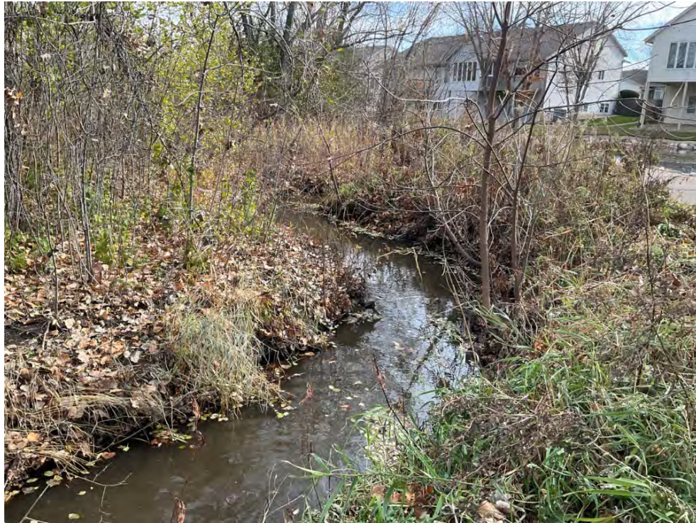
Photo 7: Site 1d. Looking downstream at station 7+75, the right bank is eroding due to a sharp turn and could encroach on the trail.
