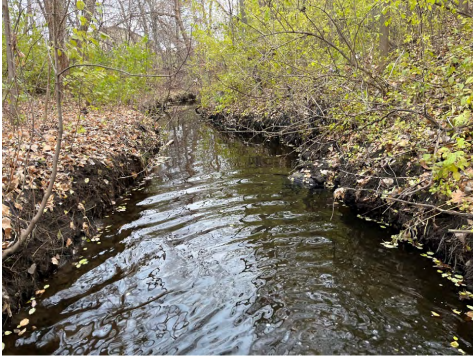
Photo 32: Site 4a. Looking downstream at station 55+00, both banks have slight undercutting at the water line.
