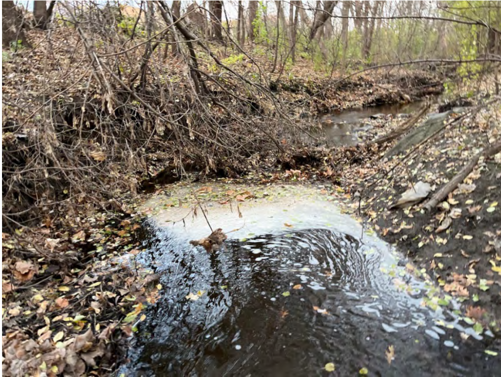
Photo 38: Site 4e. Looking downstream at station 63+00, mild channel blockage.
