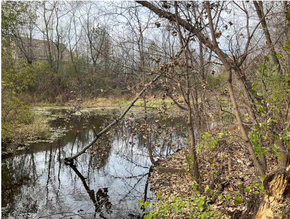
Photo 18: Site 2b. Looking upstream at 23+20. Roughly 40% of the channel width is filled in. Most of the sediment buildup is 1 foot above the water surface level, with a few locations reaching 2 feet higher than the water surface.
