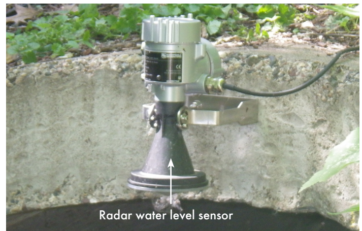
Figure 2 Radar water level sensor
