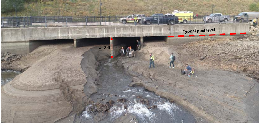
Figure 6-3 Sediment Accumulation at Tunnel Outlet
