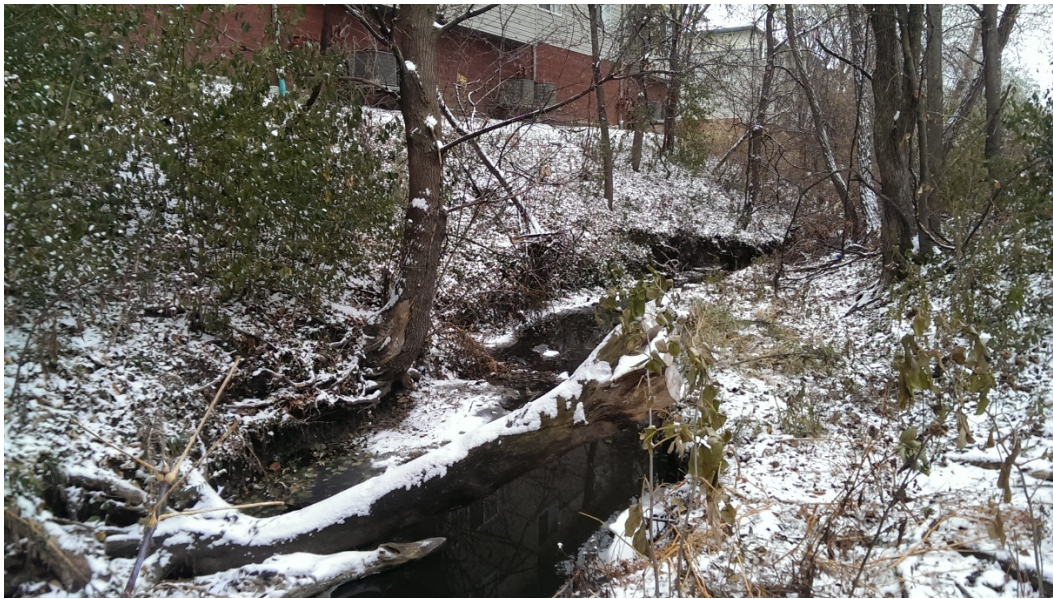
Figure 26 – Parkers Lake, Reach 1, undercut bank and bank scarp erosion
