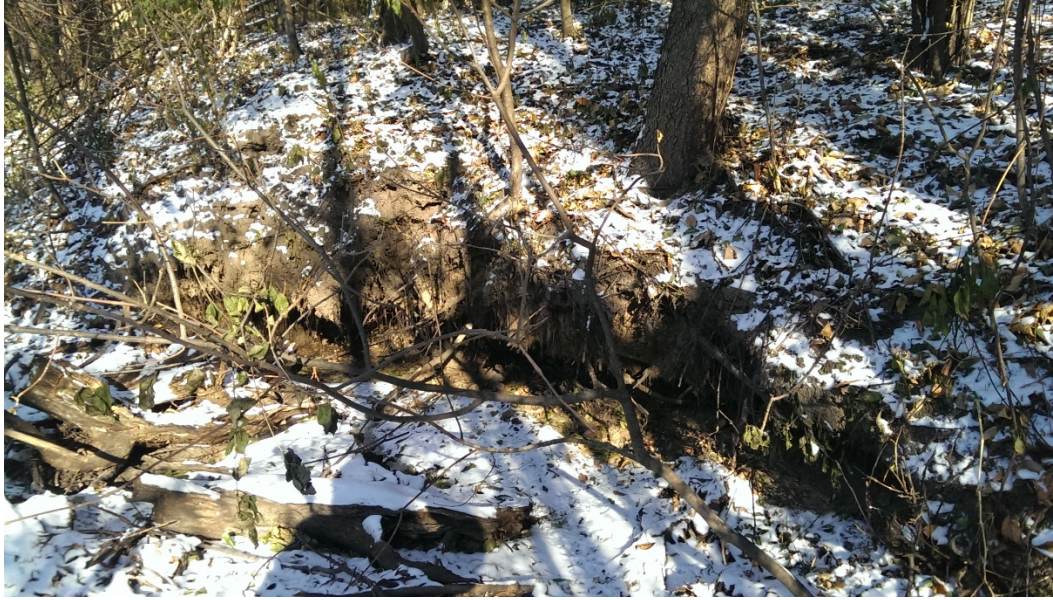
Figure 5 – Mt. Olivet, Reach 2, undercut bank and bank erosion caused by debris in channel (zoomed in location of previous figure)
