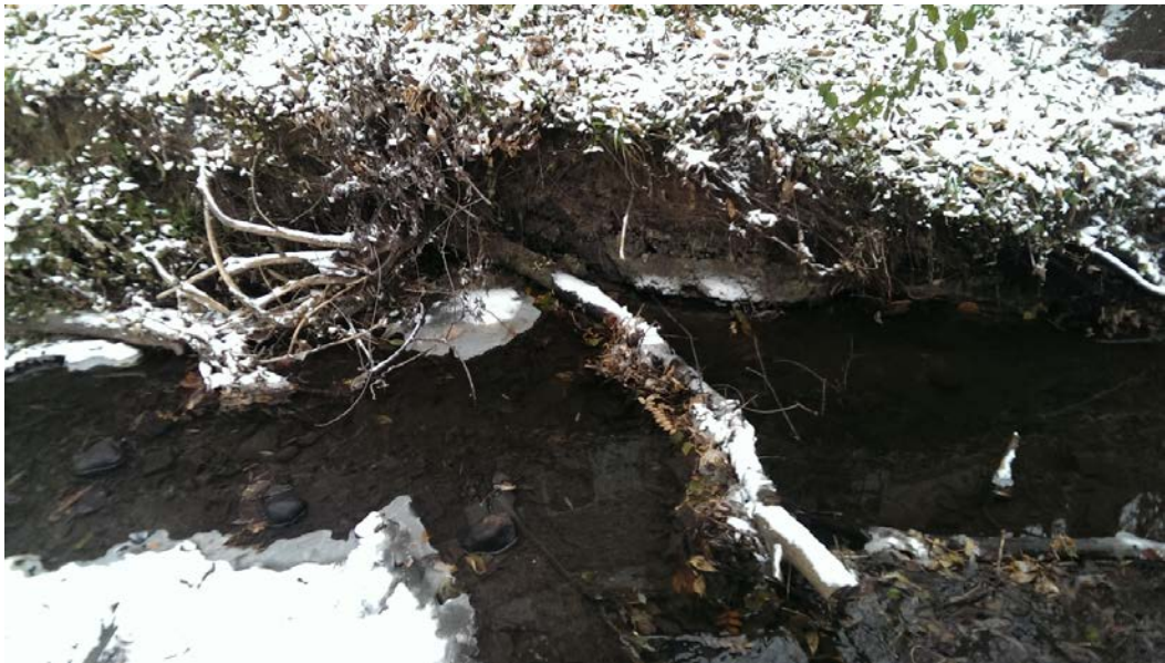
Figure 31 – Parkers Lake, Reach 1, undercut bank and bank erosion (zoomed in of previous figure)
