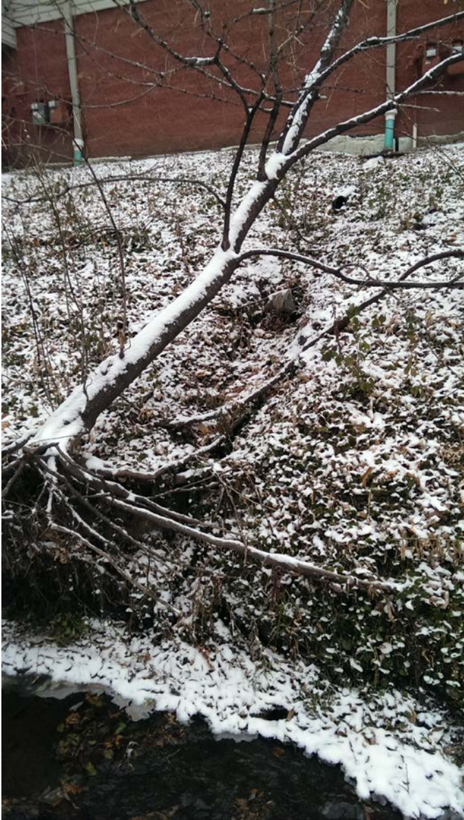
Figure 29 – Parkers Lake, Reach 1, slope erosion caused by runoff from apartment drainpipe
