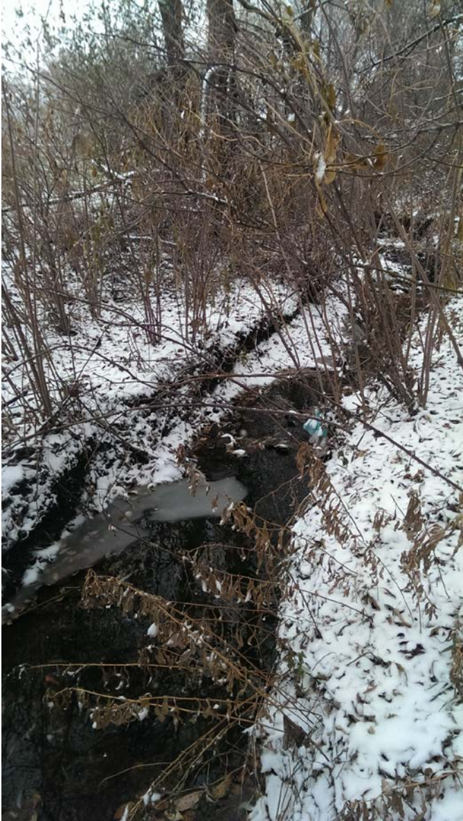
Figure 36 – Parkers Lake, Reach 1, bank erosion
