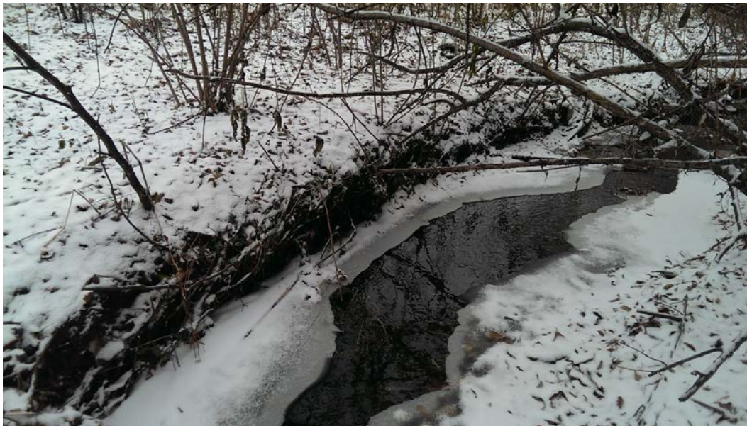
Figure 35 – Parkers Lake, Reach 1, bank erosion
