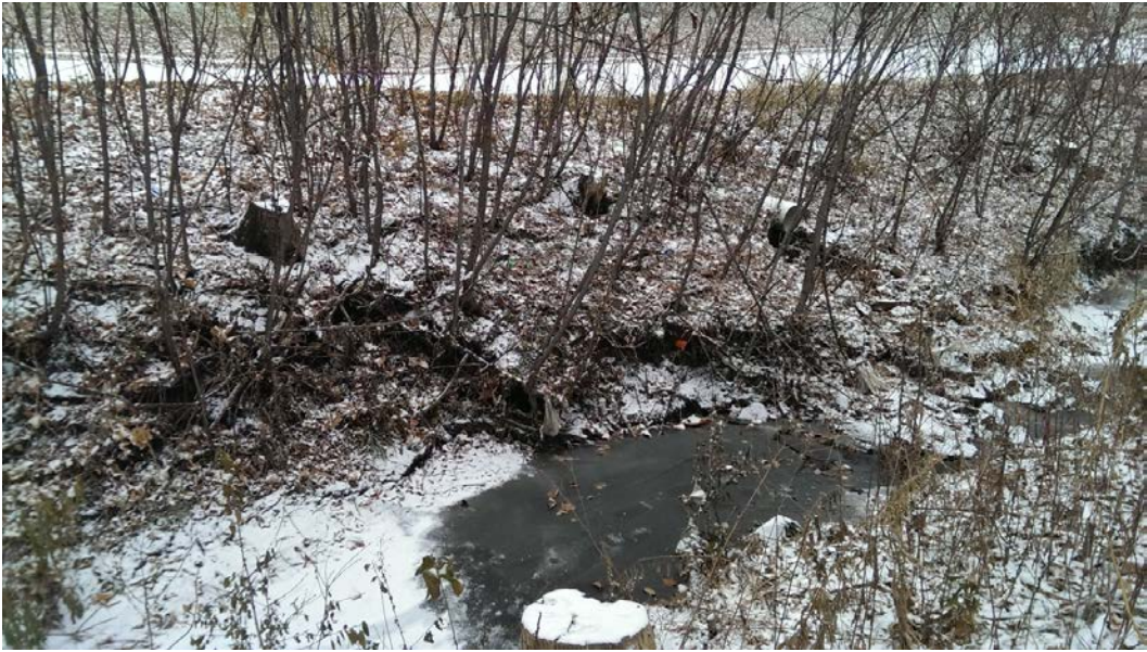
Figure 38 – Parkers Lake, Reach 2, bank scarp erosion
