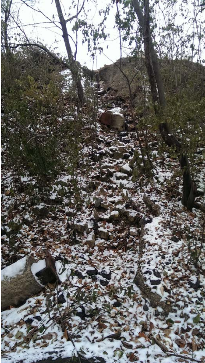
Figure 13 – Mt. Olivet, Reach 2, slope erosion from parking lot down to the stream (view from below, same location as previous two figures)
