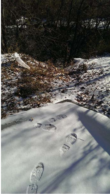
Figure 11 – Mt. Olivet, Reach 2, slope erosion from parking lot down to the stream (view from above)
