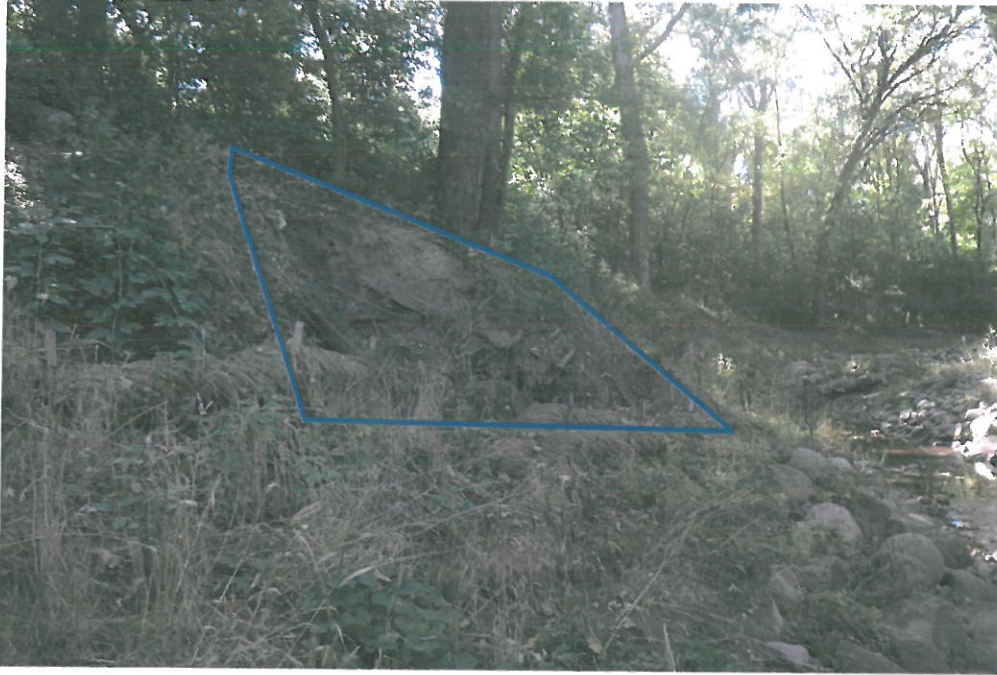
Photo 1. Upstream erosion location. Purple box shows slope erosion upstream of oak tree.
