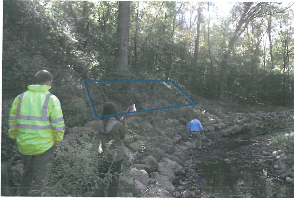
Photo 2. Downstream erosion location. Purple box shows erosion above riprap.
